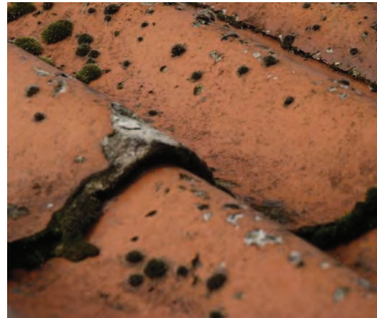
Friable roof surface (4.14)
